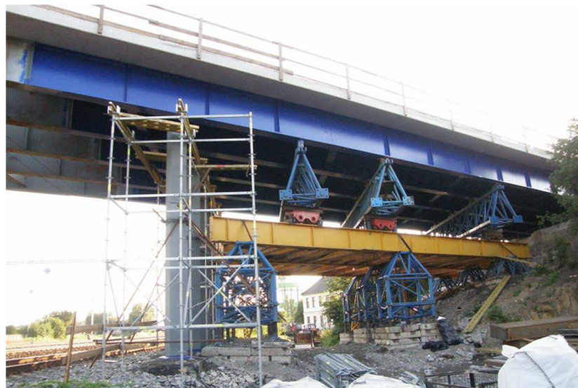
Fig. 3 – Partly repaired bridge before collapse
