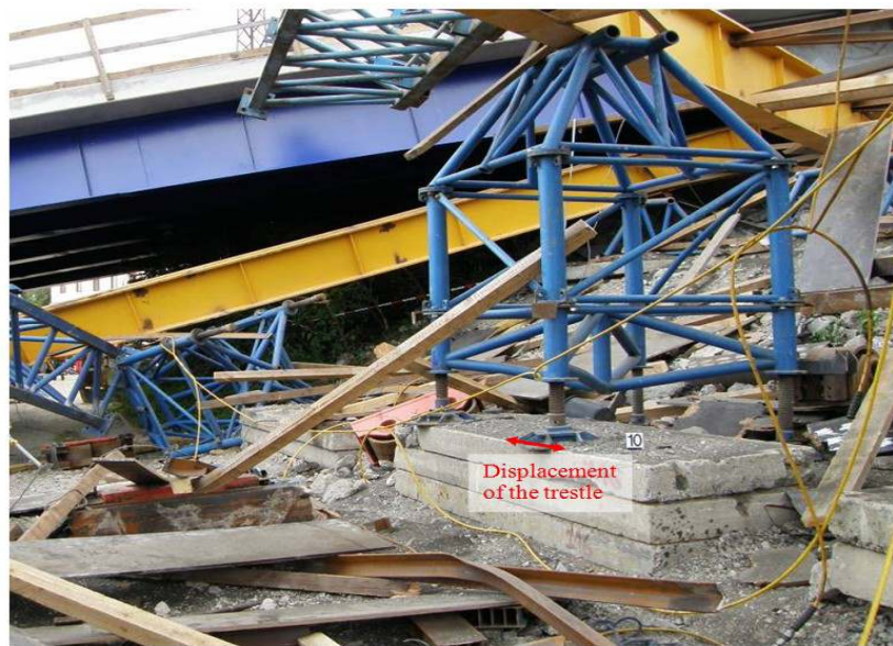
Fig. 4 – Critical trestles after collapse
